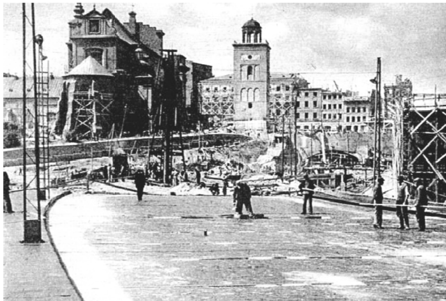
Fig.2. View of the St. Ann's Church during the construction of Warsaw's East-West Route in 1949 ( origin PAP )
