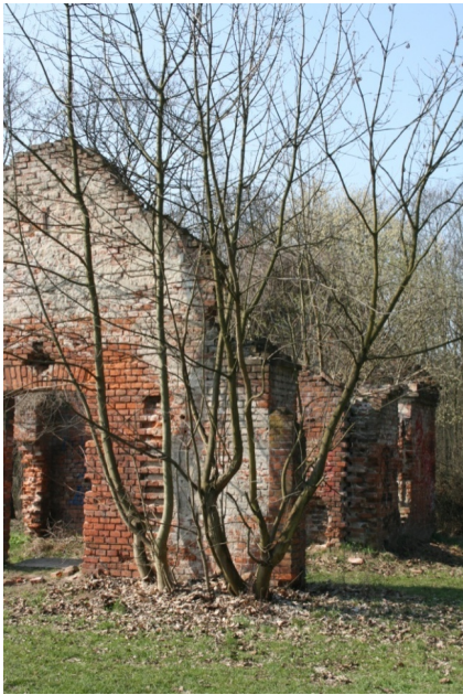
Figure 2. Ruins of the Cracow Fortress in Wola Duchacka – visible front and north elevation. (March 2025, phot. A. Malec)
